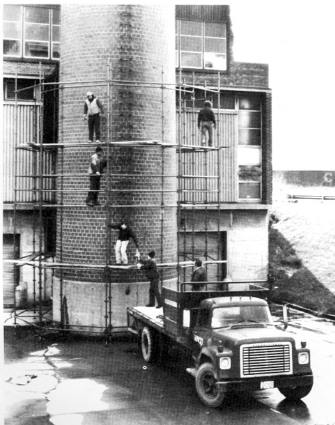
CIRCULAR OBJECTS — chimneys, structural columns and other objects of any size with a consistent diameter.
